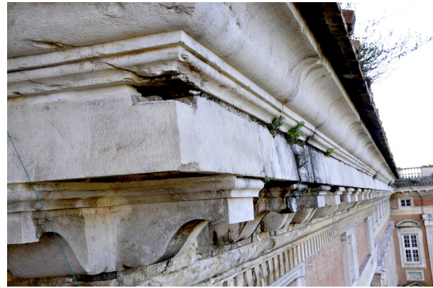
Fig. 1 Before restoration: degradation of stone mouldings caused by rain water.
